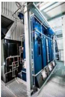
Sistemul de alimentare (HOST Bio-energy installations)
