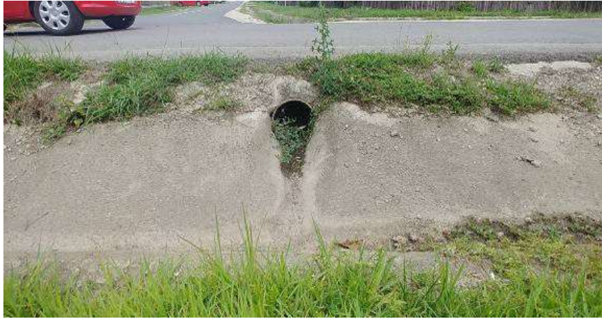
Fig. 3 . Podet drum latereral partial colmatat km 0+192
