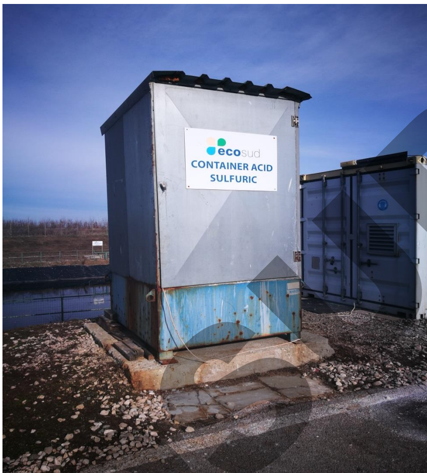
Figura 24. Container acid sulfuric
