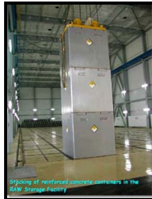
Figure 5 Reinforced concrete containers for disposal of RAW in the NDF
